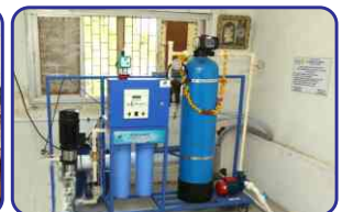
Clean Drinking Water
